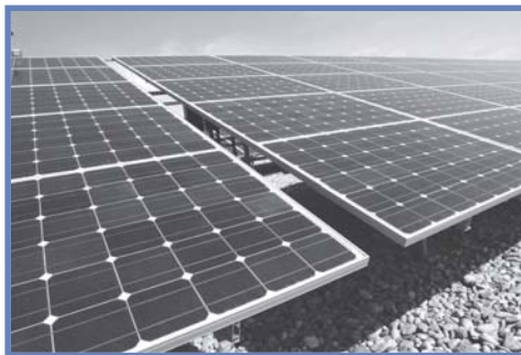
A solar panel array. Typically, a smaller setup would need only a few panels (or a single medium sized panel) to fulfill some of its energy needs.
